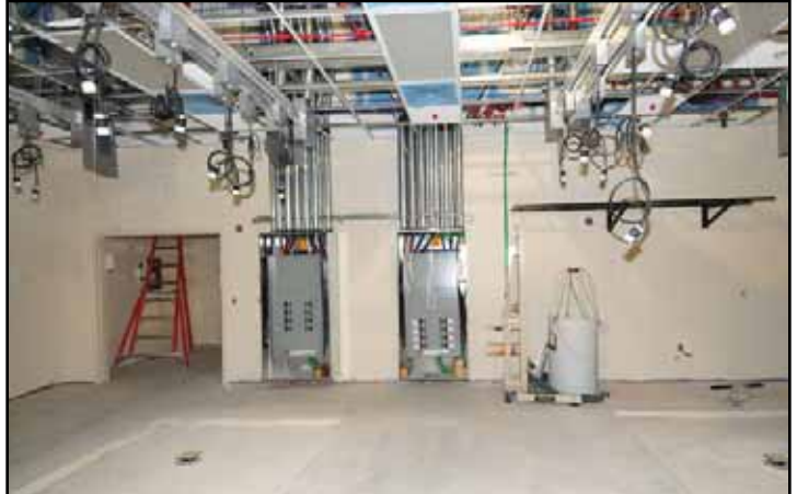
Electrical panels inside the Clinic Building North data center.
