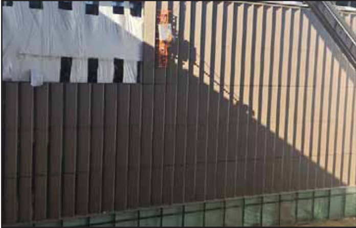
Exterior curtain wall on the east facing zig zag wall of the Concourse between DAT and IBS.
