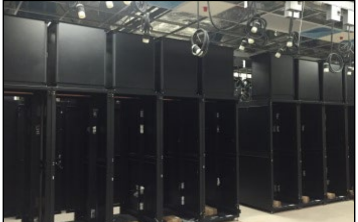
Server racks installed in the Clinic Building North data center.
