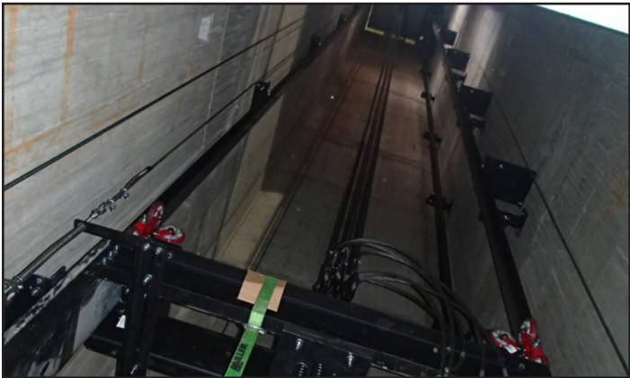
Elevator shaft equipment placed in the Research Building.
