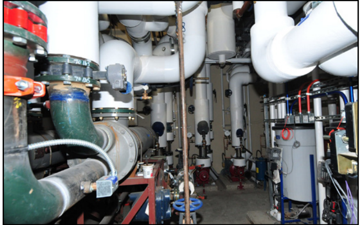
Mechanical equipment in the Inpatient Building South Penthouse.
